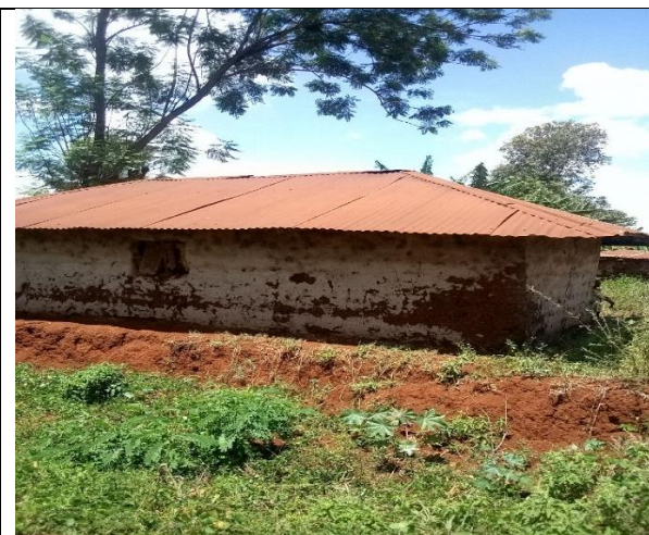
Figure 15: Vulnerable PAP Housing structure
