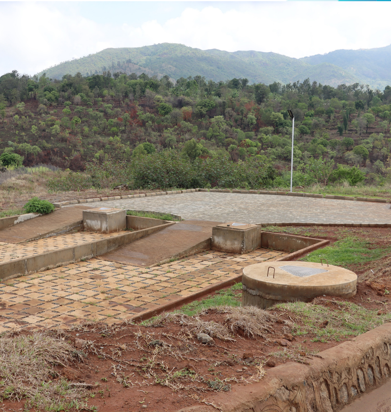
Chogoria SEwerage - Sludge Drying Beds
